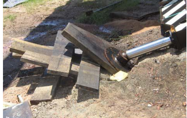
Photograph 2: Example of consequences of poor ground and inadequate support
